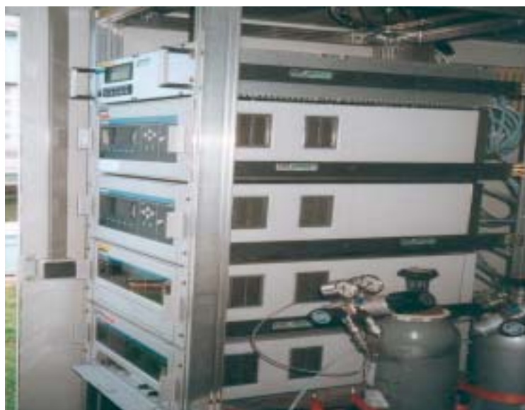
The interior of the mobile measuring station
